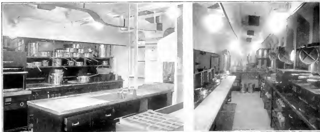
General-Electric illumination gives daylight effect in the galley and pantry on the steamship Escalbur.
